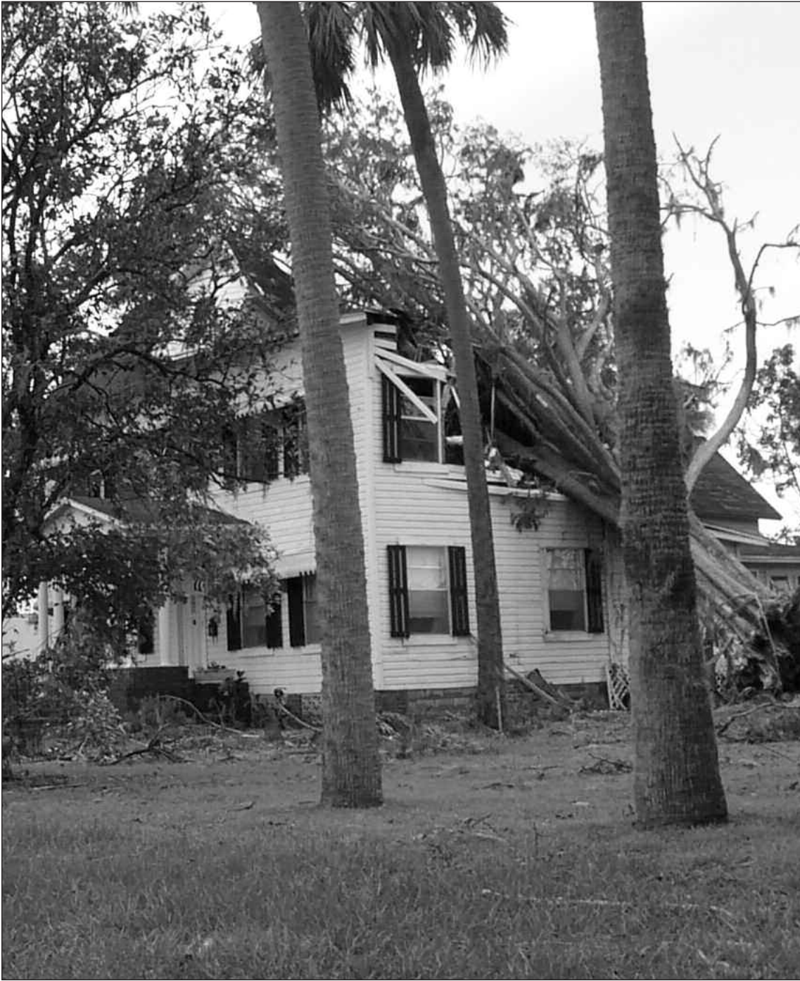
Even substantial and well built homes in Wauchula, FL were victims to the violent winds of the hurricanes. There was no respect shown by the storms for anything the stood in their way.
