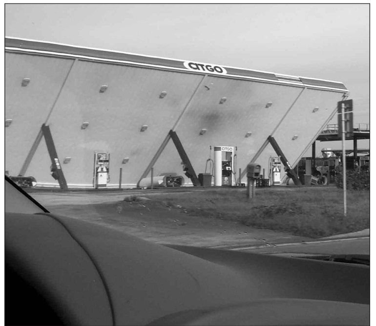
The Citgo Station in Bowling Green, FL lost its canopy.
